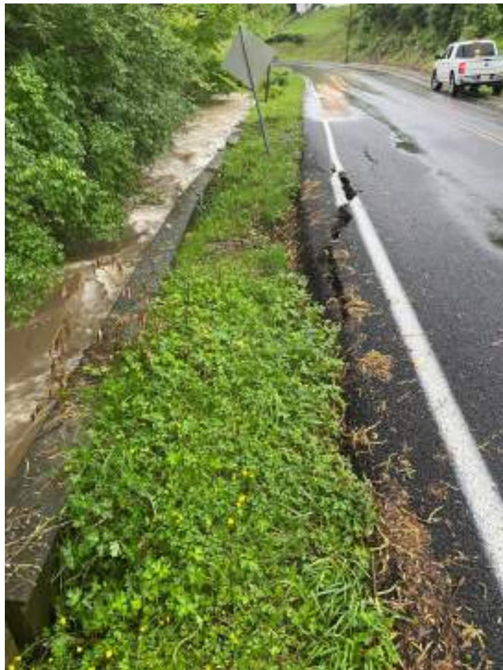
Figure 645: Road Damage in Bluefield, VA from Flooding in March 2023
